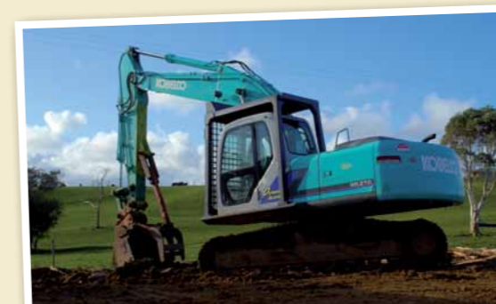
THE SMITH'S ISOLATION MEANS THEY NEED TO BE COMPLETELY SELF-SUFFICIENT WHEN IT COMES TO PLANT AND EQUIPMENT. THEY EVEN HAVE THEIR OWN EXCAVATORS.
